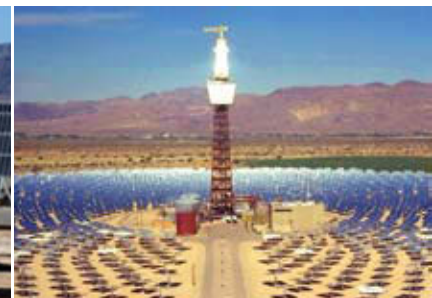
Concentrating solar power tower – courtesy Sandia National Laboratories
