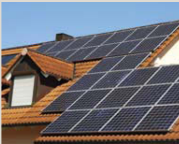
Home solar power
